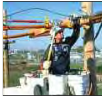
Insulated for Electrical Work*
